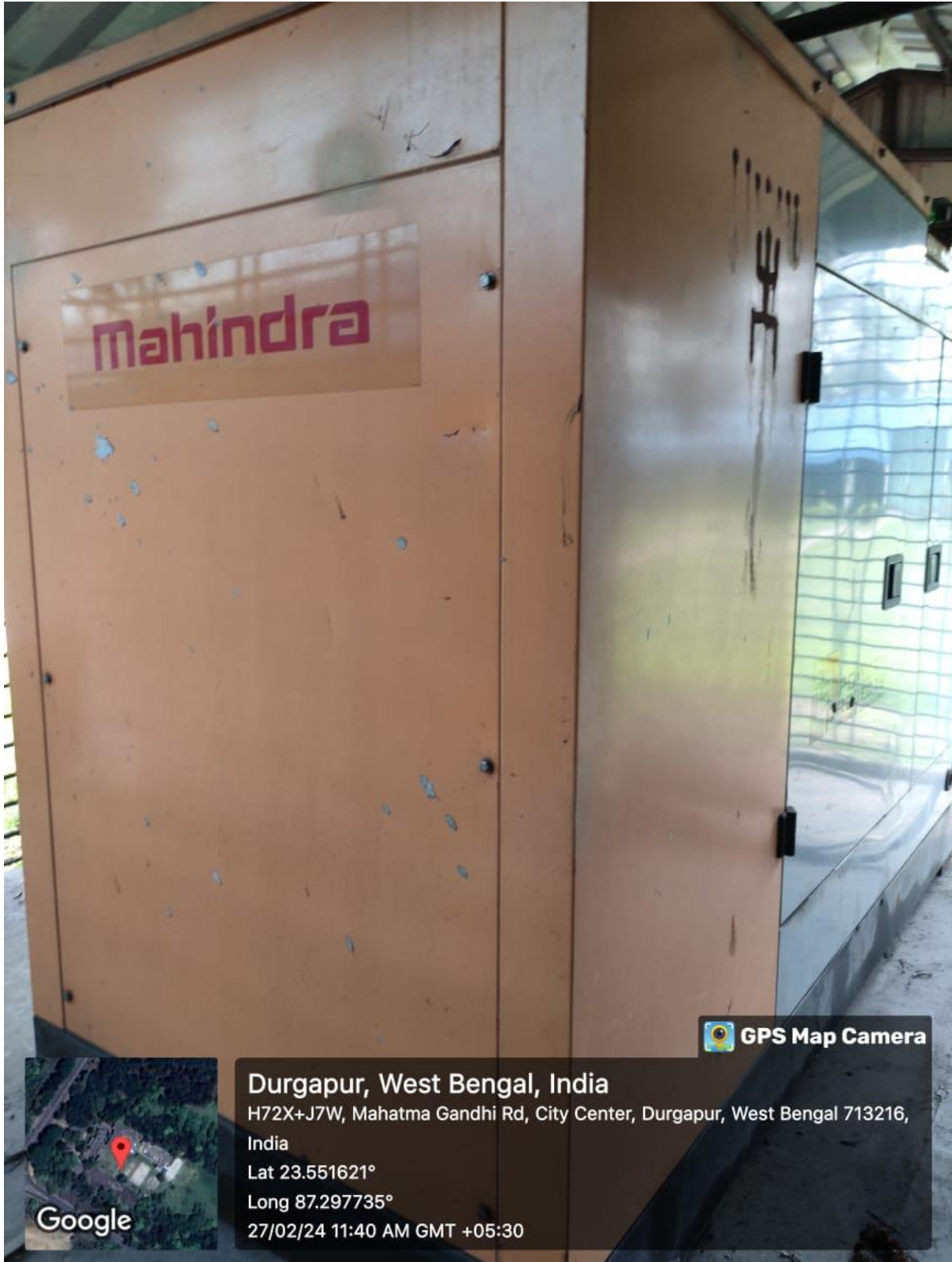
Power and Fuel Efficient Green Generator
