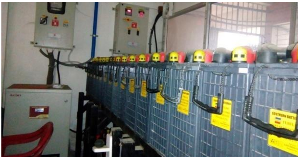
The Solar Power System
